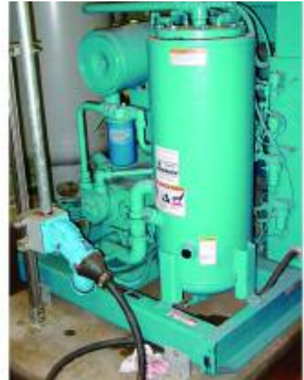
Primary Air Compressor
