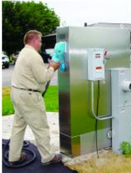
Remote Lift Station
